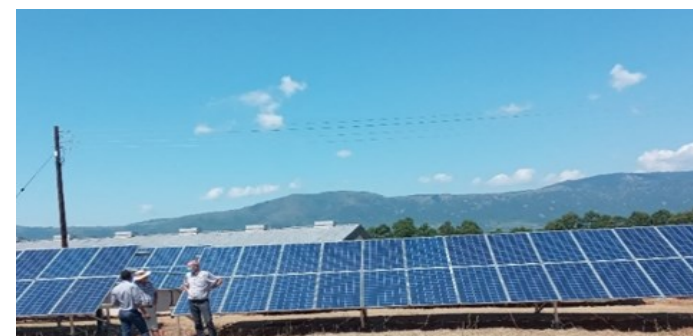
Figure 3: Solar panels in one farm in the Malkerns area
