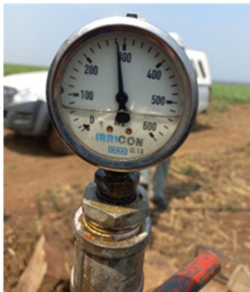
Figure 2: A pressure gauge showing pressure reading from a hydrant valve
