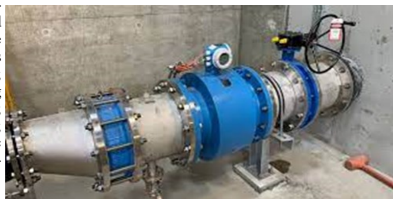
Figure 3: A flow meter installed in an irrigation pipeline
