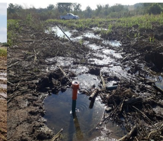
Figure 3: Leakage leading to drainage problem
