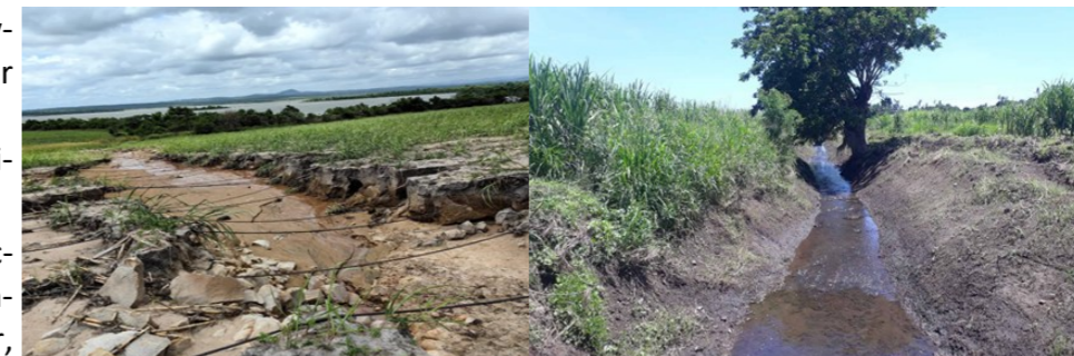
Figure 3: Severe soil erosion due to lack of proper storm water drains (left) and a properly maintained stormwater drain (right).
